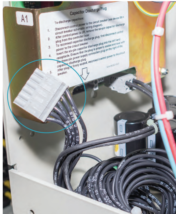
Detail of electronic controller and pull to discharge capacitors
