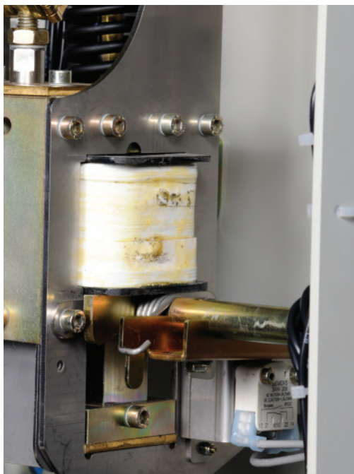
Interlock not blocked (cover removed for photo)
